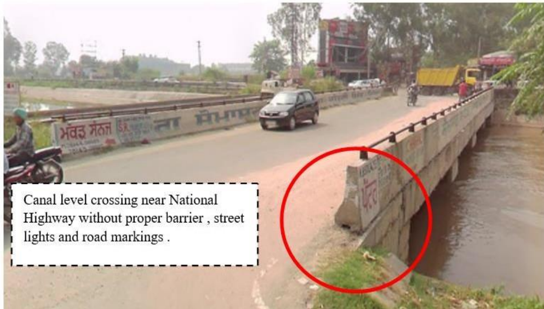
Figure 3.15 Observed problems highlighted in red
